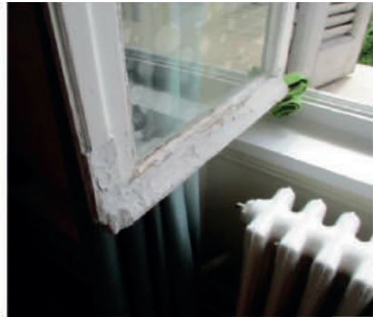
Poor historical repairs
