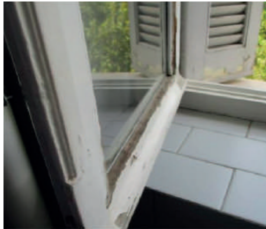
Putty missing from glazing
