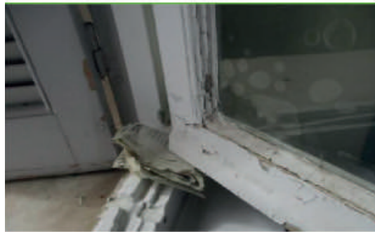
General overall decay
