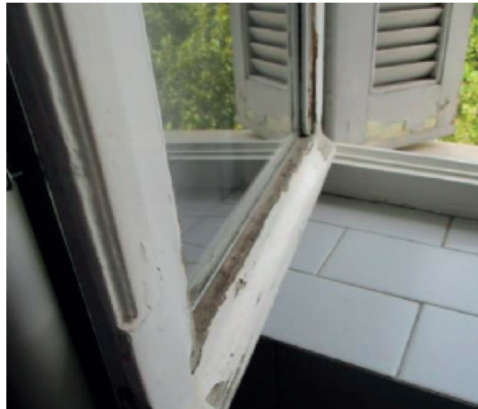
Putty missing from glazing
