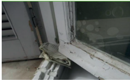
General overall decay
