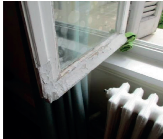
Poor historical repairs
